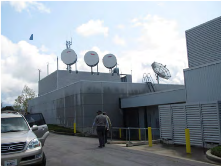
Microwave dishes at EOC network core and test server location
