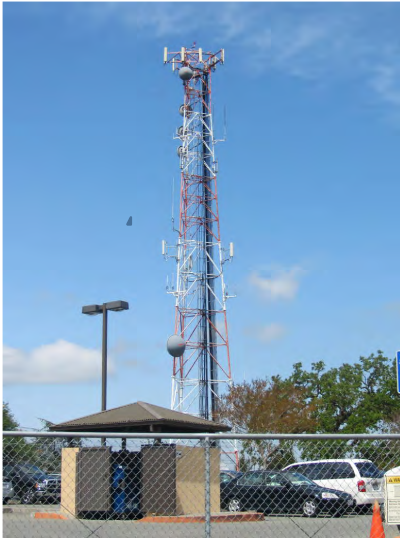
LTE Antenna location at the Glacier Street site
